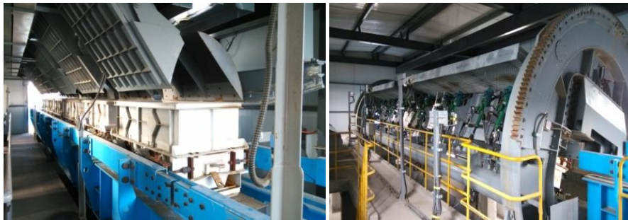
Fig. 12 Load Station (left) and Unload Station (Right)
